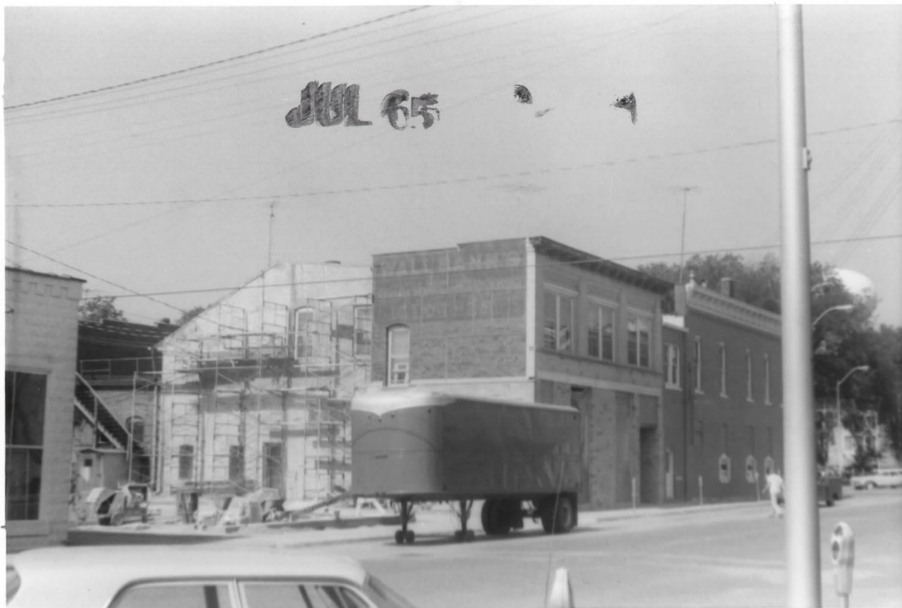
Rear of bank in July 1965 with work for drive-in bank underway and portion of building along E. Monroe St, looking southwest from E. Monroe St (HCHT collection)
