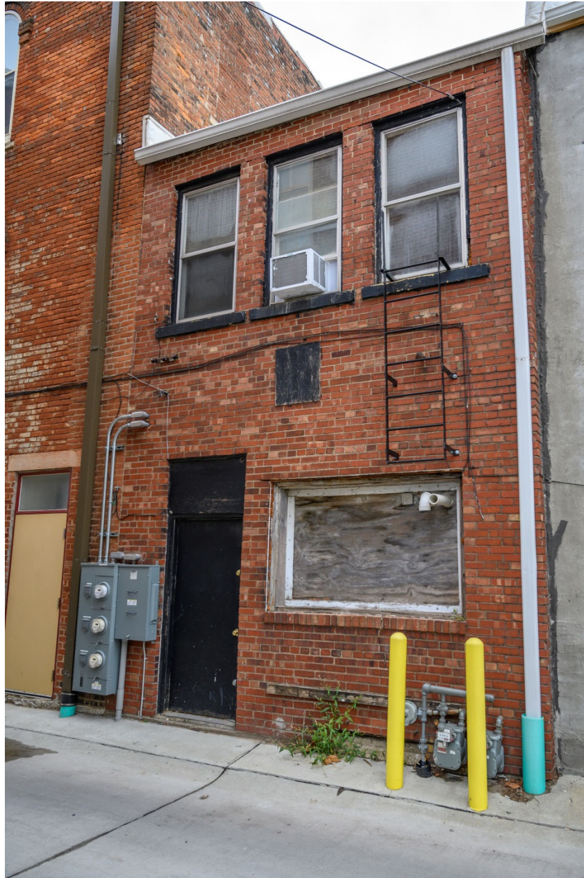
Photograph 44-00370-003. East elevation of rear section that extends east to midblock alley, looking west (October 2023)
