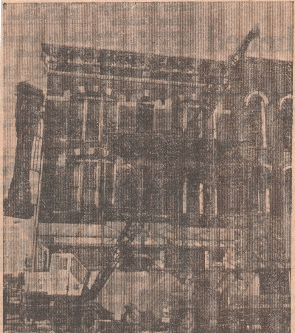
MT. PLEASANT FACE LIFTING. The Hayes Insurance Co. building in downtown Mt. Pleasant is literally "flipping its lid." The top story of the 100-year-old building at the northwest corner of the square, is being removed as part of an exterior remodeling project.
