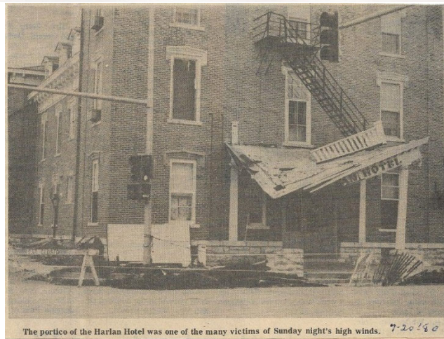
Damage to Harlan Hotel portico in July 1980 (HCHT files)
