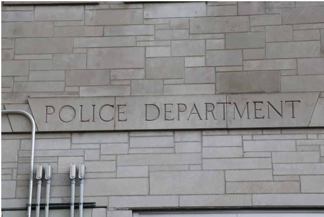
Photograph 44-00377-008. Detail on rear section of west elevation of City Hall, looking east (October 2023)
