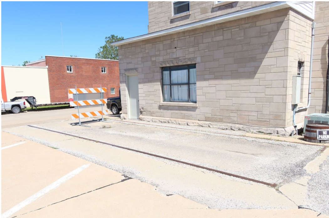
Photograph 44-00377-011. Remnants of scale south of City Hall, looking northwest (June 2024)
